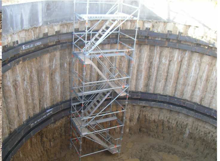
Sheet of piles 55 cm in diameter, that encloses a cylindrical working shaft, 12 m diameter, 13 m depth
