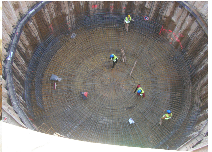
Reinforcing steel placement for the construction of the foundation slab, 1.5 m in thickness.
