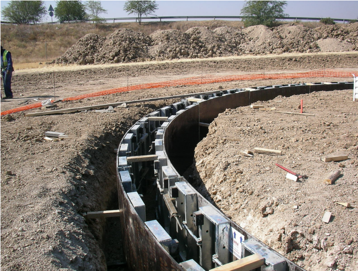
Guide beam to set out the position of the sheet pile wall
